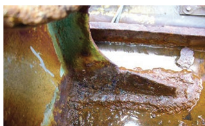
Cracked bulwark stay
