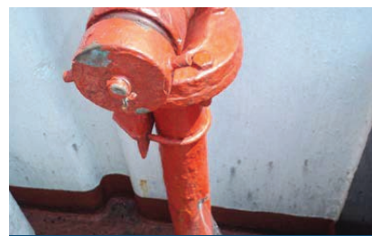
Leaked fire line
