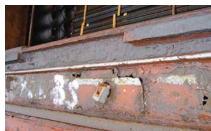
Wasted hatch way
