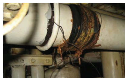
Patched sea water pipe
